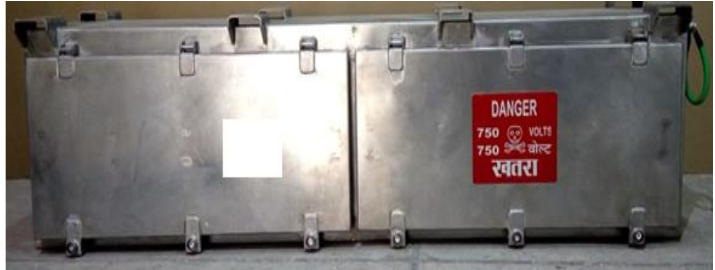
FRONT VIEW OF UNDERSLUNG SOP-355 REV-1 HV PANEL
